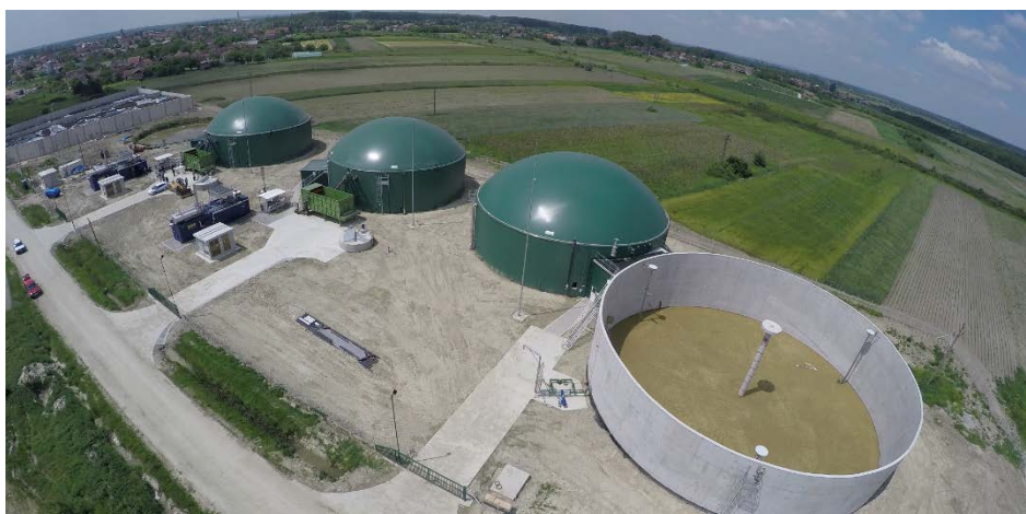
Photo I.17 Biogas CHP Plant in Bac: Aerial View of Digesters, Feeders, Biogas Storage, Engine Containers, and Transformers
