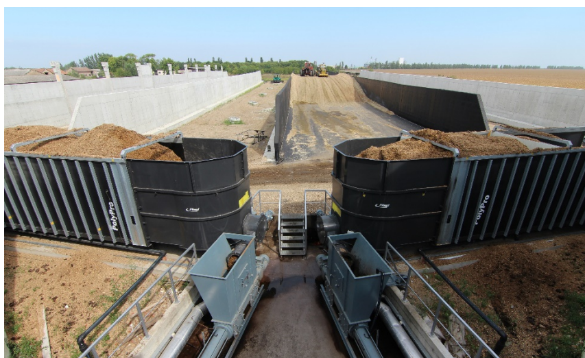
Photo I.18 Biogas CHP Plant in Alibunar: Trench Silos and Biomass Feeders
