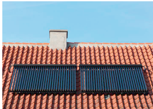
Active solar system with vacuum-tube collectors
