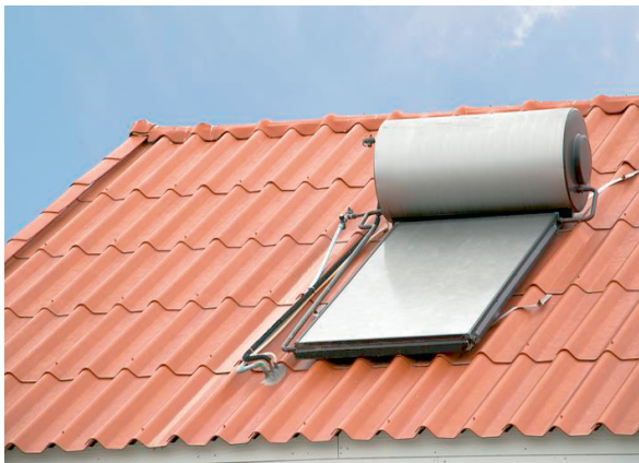
Passive solar system with flat collectors
