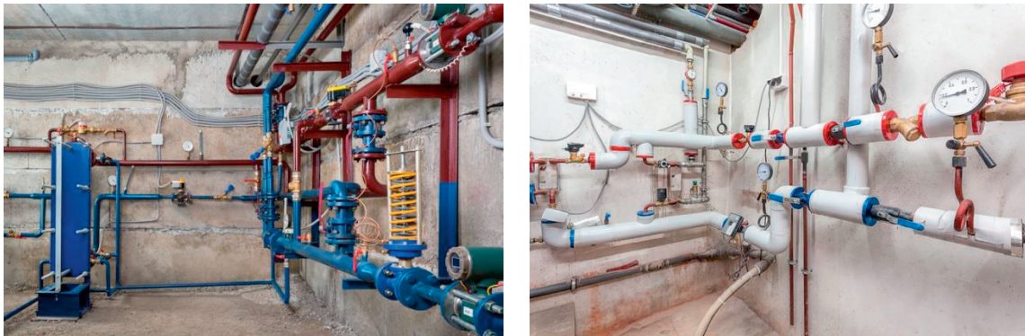
Figure 8. Individual automatic heat point with weather compensation control
