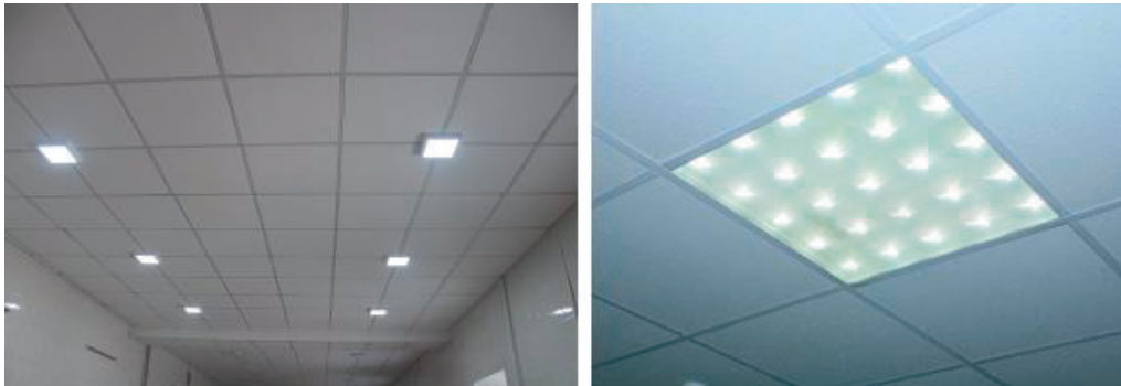
Figure 15. Light-emitting diode fixtures
