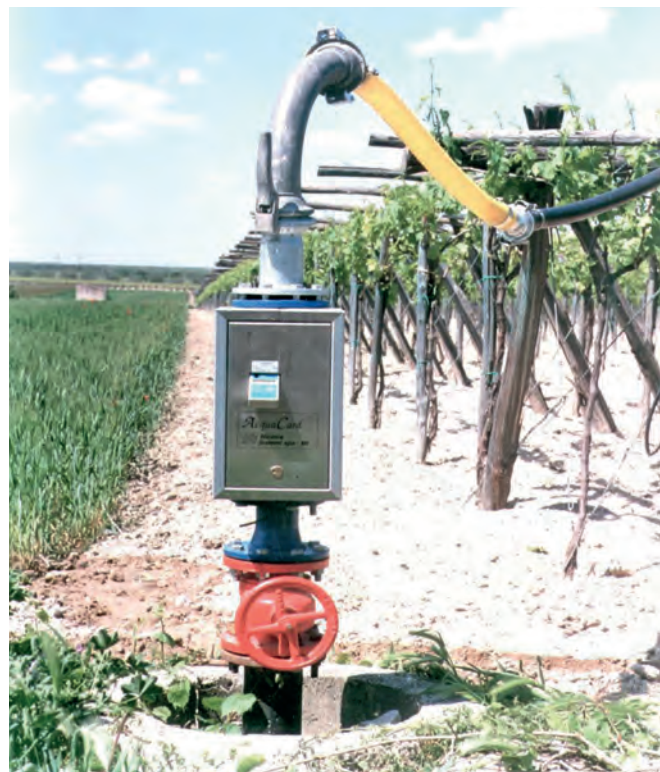
Irrigation hydrants for automatic, selective and controlled water distribution, equipped with a hydraulic device coupled with electronic components. The quantity of water supplied can be programmed by an electronic card assigned to farmers
