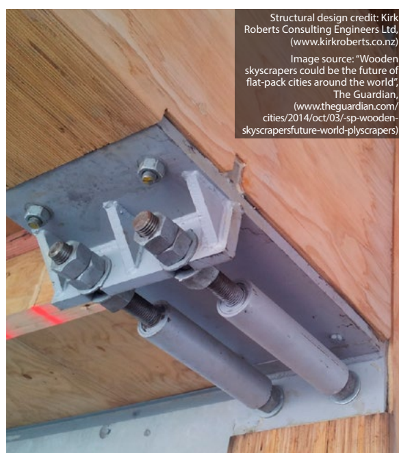
Figure 27: Detail of the Merritt building in New Zealand is the first post-tensioned wood frame building designed to withstand extreme seismic events
