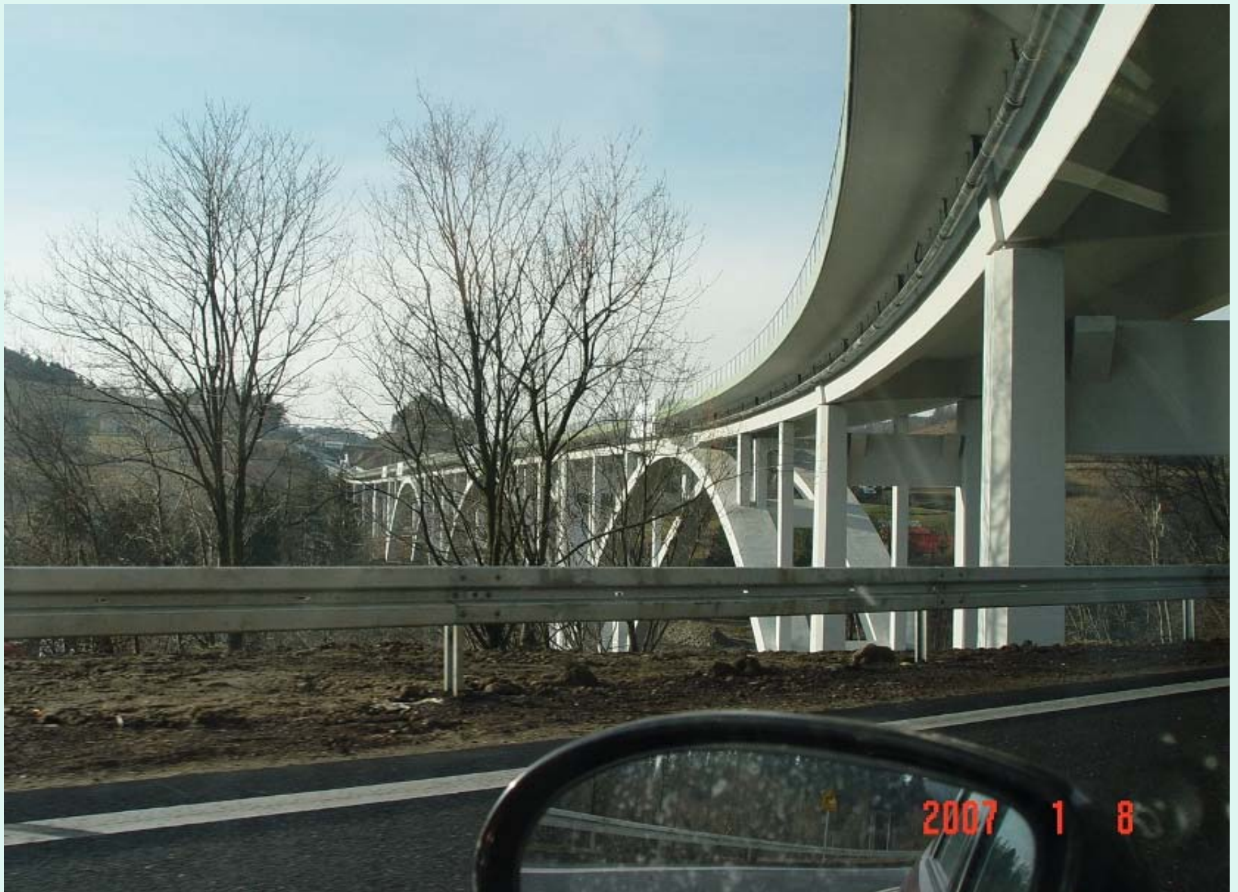
Newly opened section of the S-69 national road in Polish section of Corridor VI (Żywiec – Zwardoń) running through an estacade along the Soła river.
