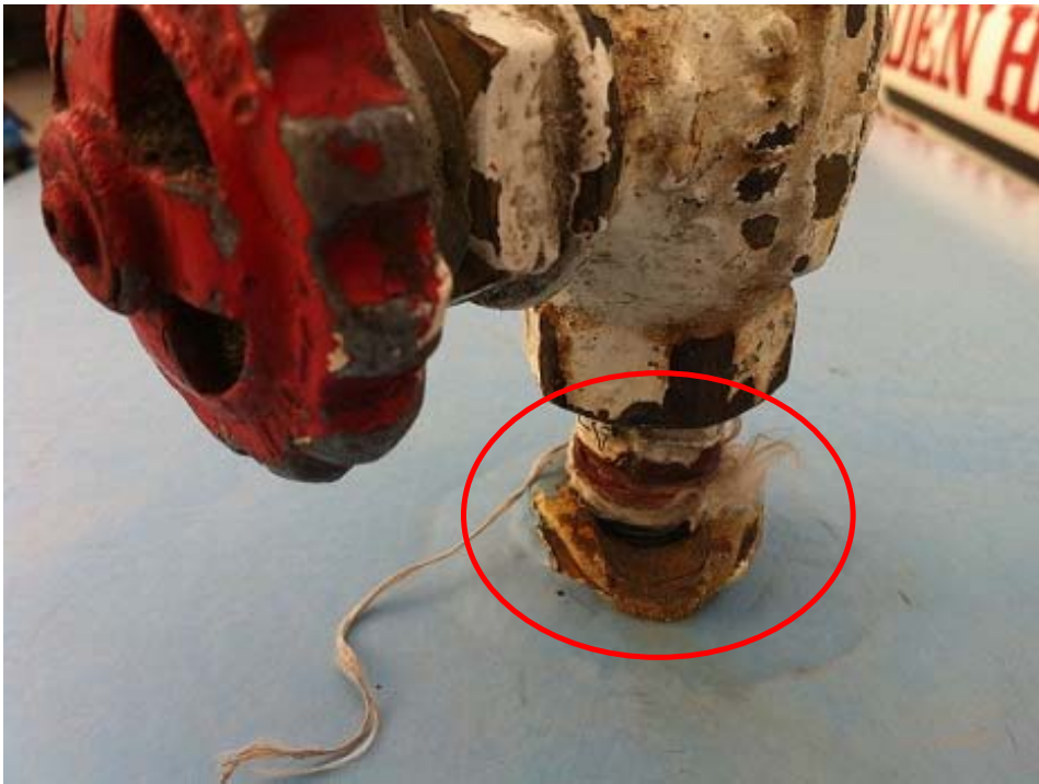
Damaged tank (after a valve was placed to contain the gas leak)
