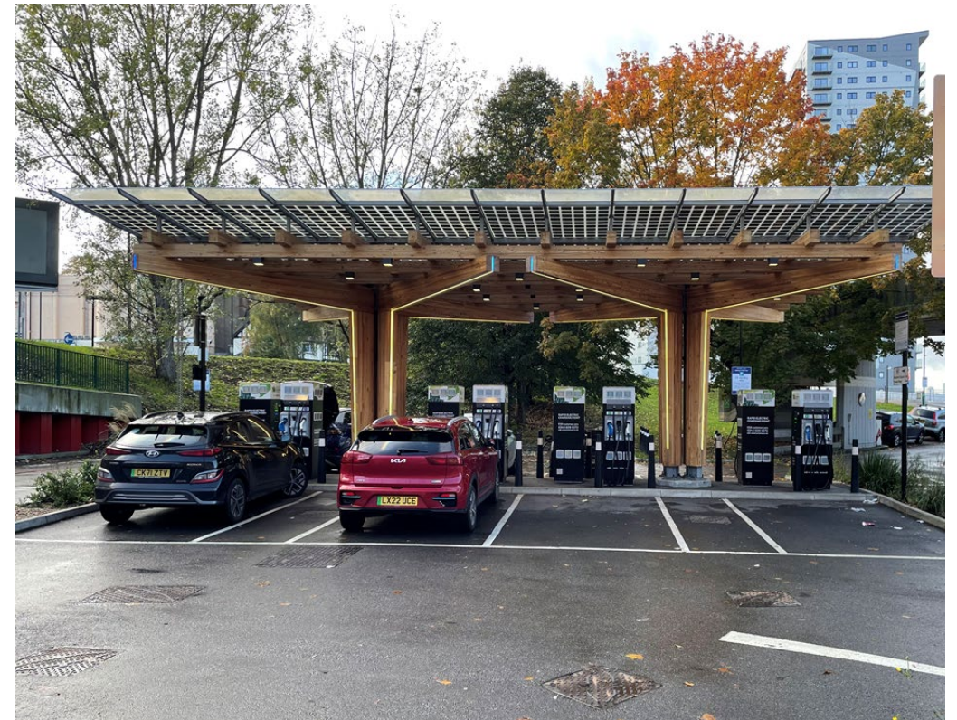
8 charging devices with 24 connectors
